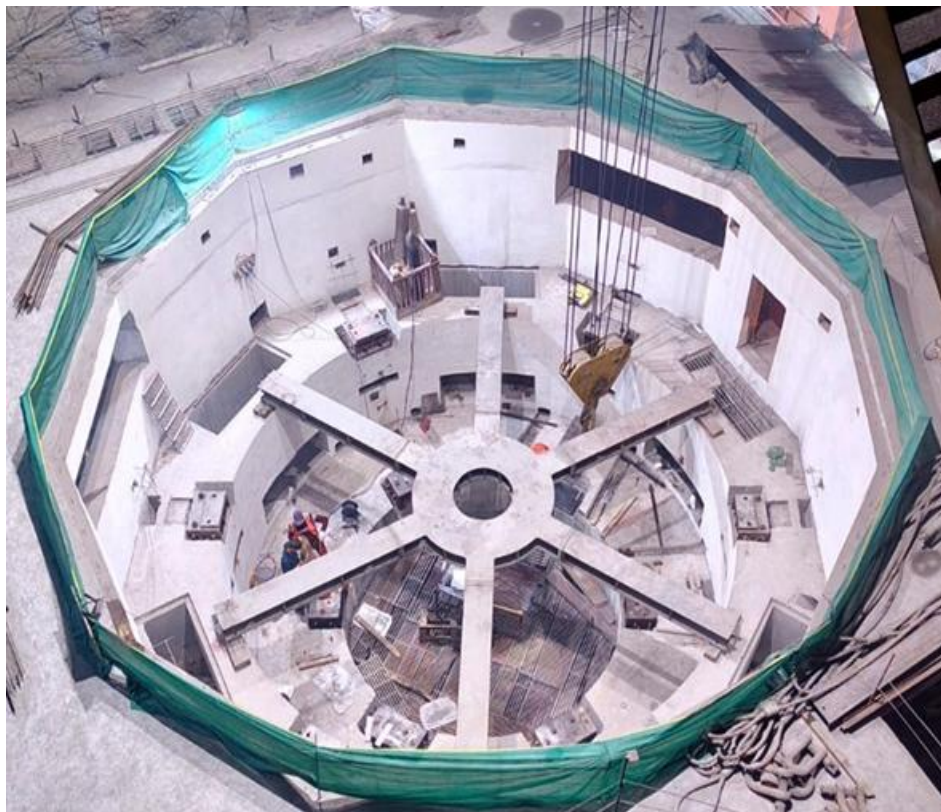
Machine Hall Unit 1
