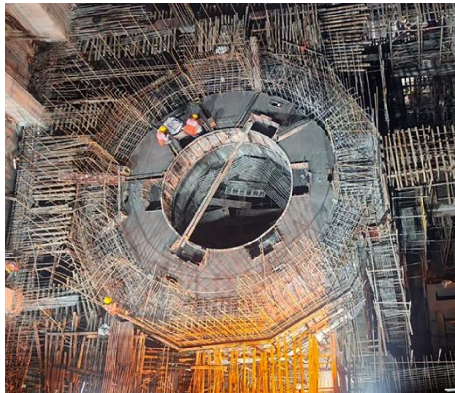
Machine Hall Unit 3
