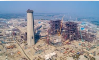
2X660 MW at Rampal, Maitree, Bangladesh-BIFPCL
