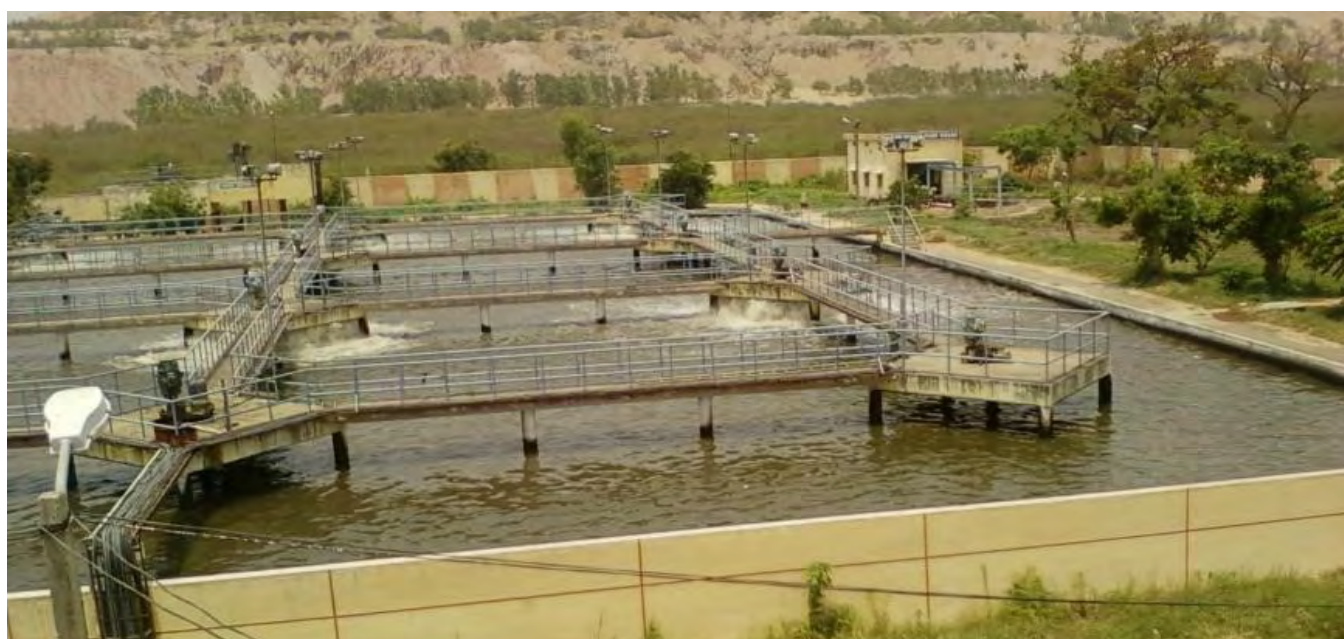
Municipal Sewage Treatment Plant – Neyveli Township
