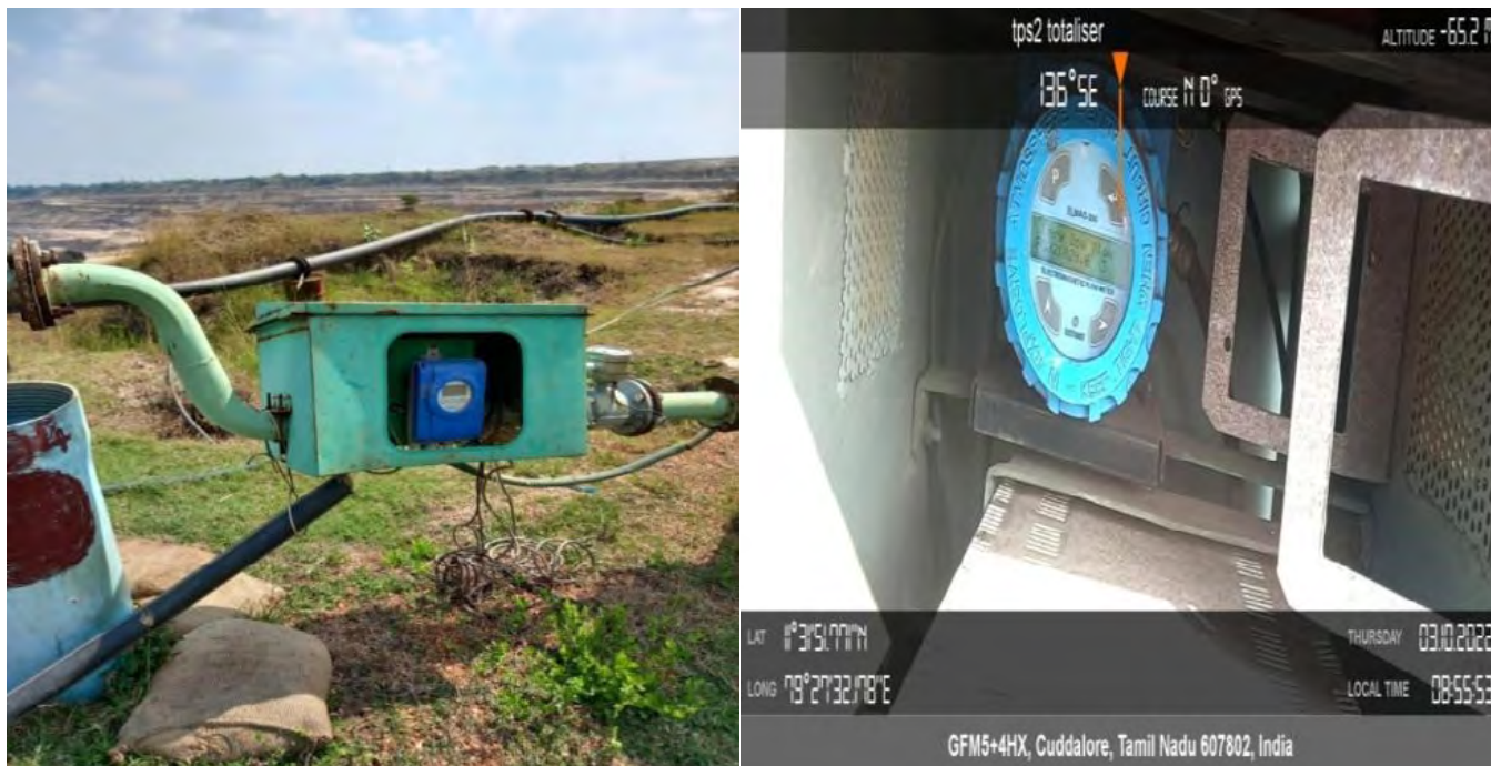
Flow Meters Installed
