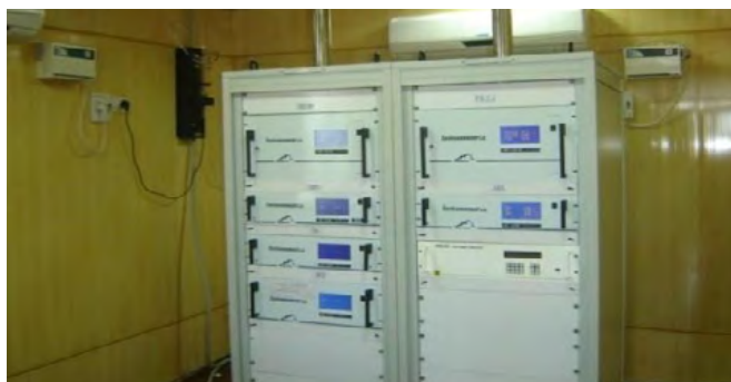
Installed CAAQM Stations
