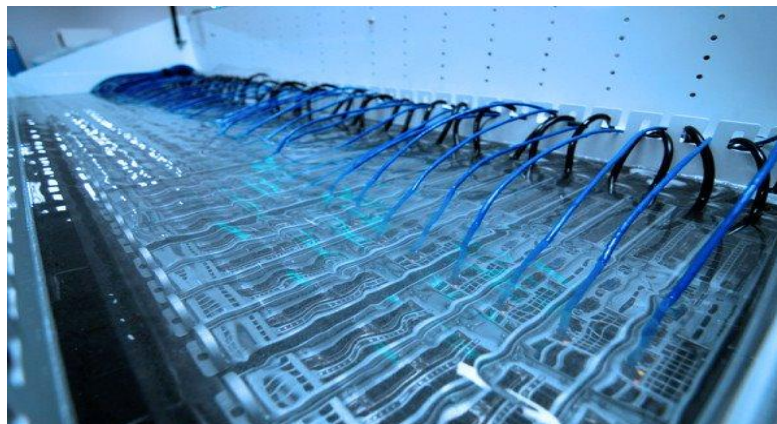
DATA Centre Cooling
