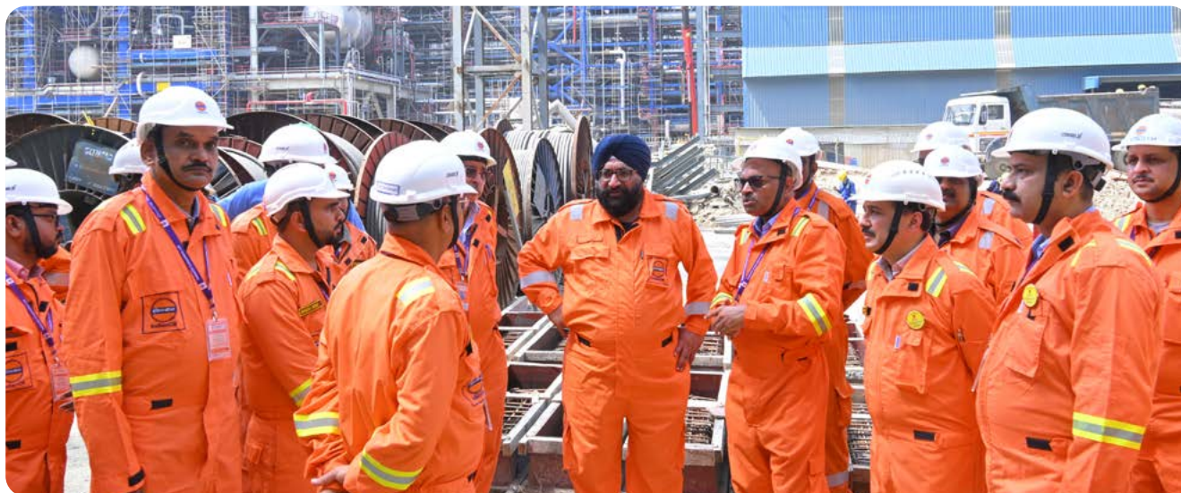
Chairman with team Panipat Refinery and Petrochemicals Complex
