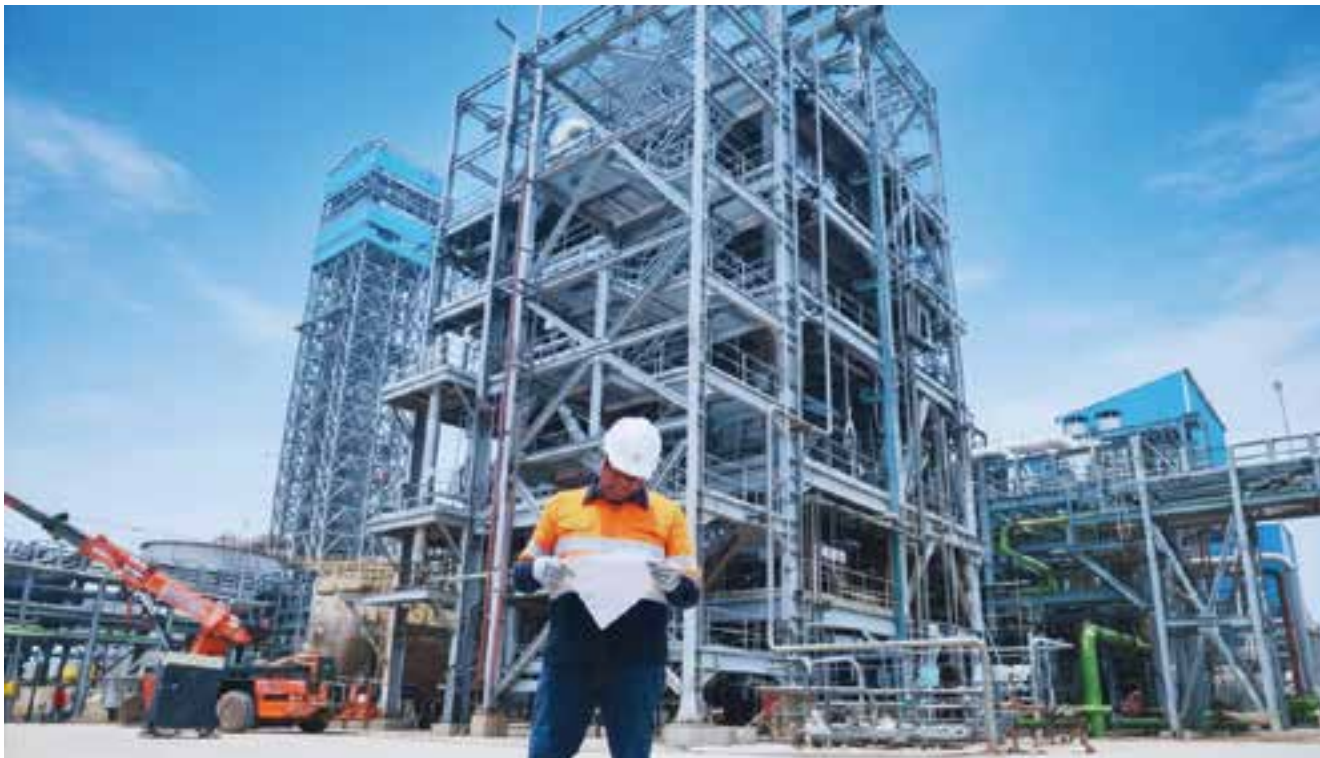
▲ Ammonium Nitrate Solution plant at Gopalpur Project site.
