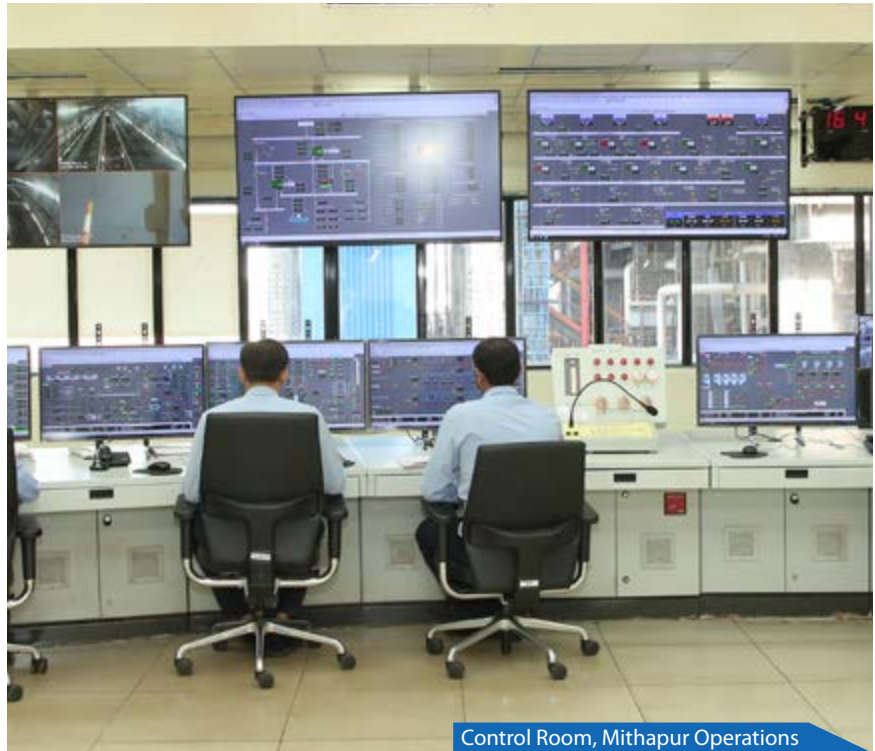
Control Room, Mithapur Operations
