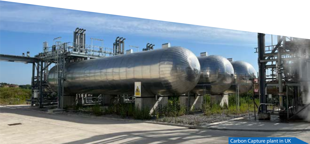
Carbon Capture plant in UK
