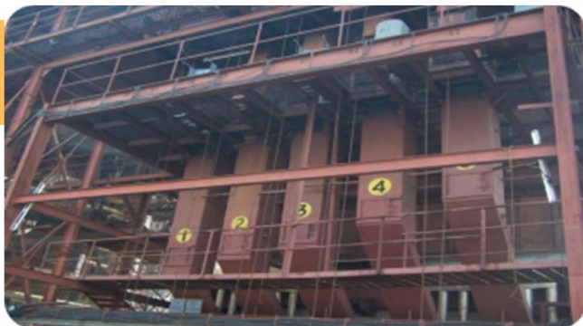
Bagasse silos & feeders of boiler
