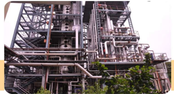
Distillation house & multi-effect evaporator
