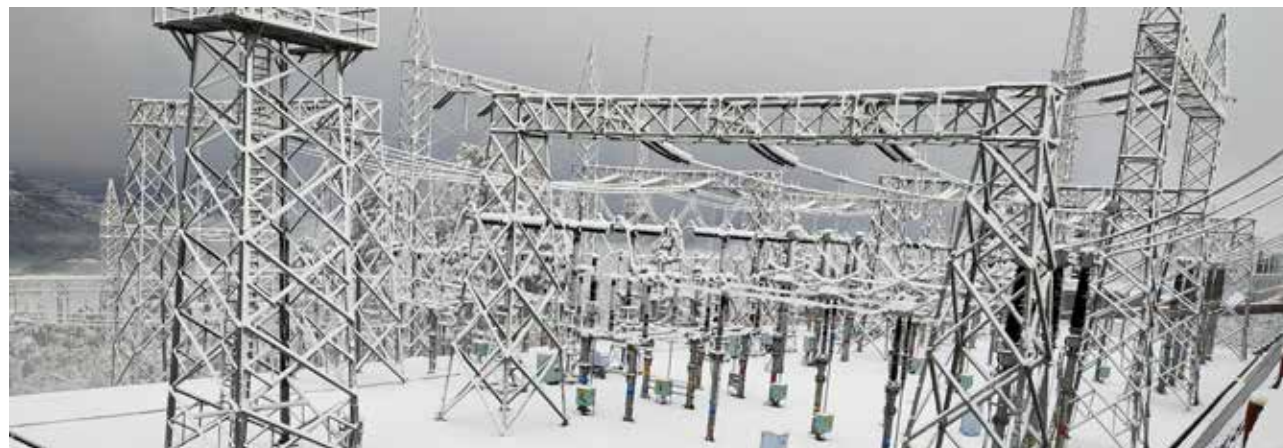
View of Pithoragarh Substation
