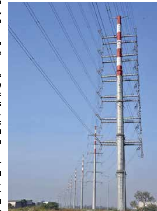
Monopole with Insulated Cross Arms
