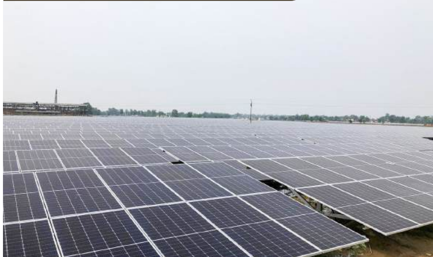
Offsite solar plant for Phoenix Palassio, Lucknow
