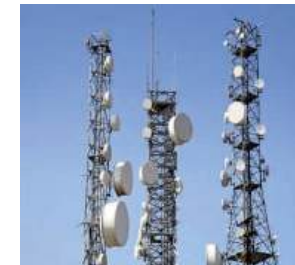
5G Telecom Towers
