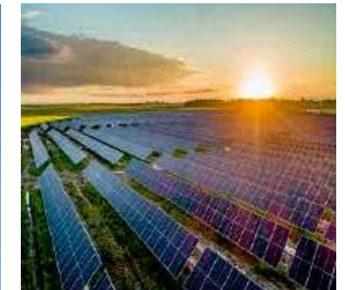
Solar Mounting Structures
