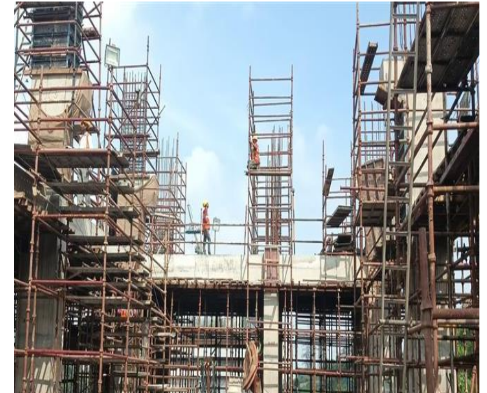
Data Center substation & line - construction of 220/33 KV GIS Substation and associated Transmission line Substation: 1 (no.) Status: On-going
