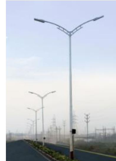
Lighting Poles & Masts
