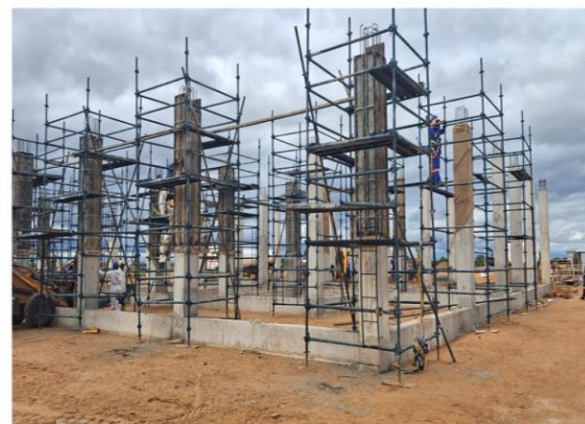
400kV Mmamabula Substation project (Botswana)
