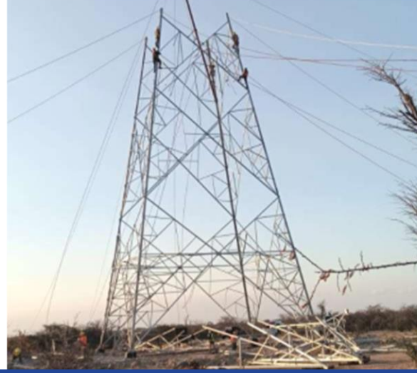
400 kV D/C Transmission Line TaZa Project (Tanzania)
