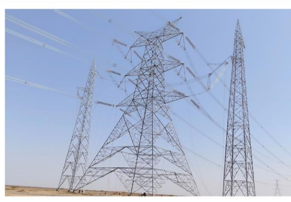
765 kV D/C Transmission lines in Khavda, Gujarat
