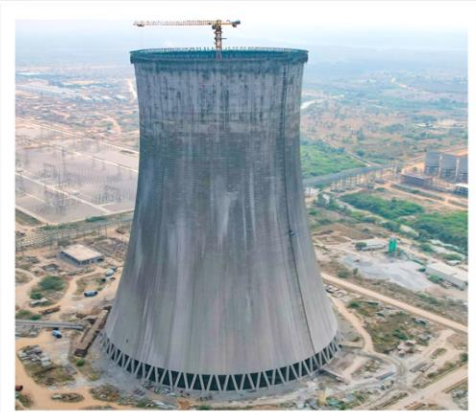
Cooling tower at Udangudi and Yadadiri
