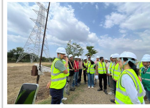
MCA-Nepal Board of Directors visited 400 kV Butwal Substation project site
