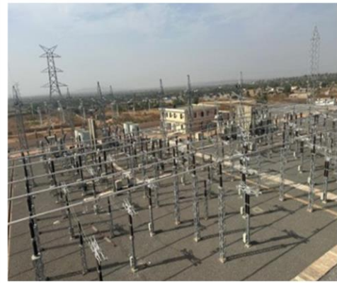
225/30 kV Substation project at Mali
