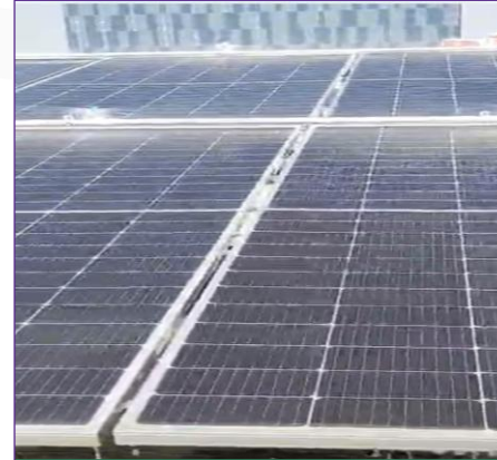
Rooftop solar installations
