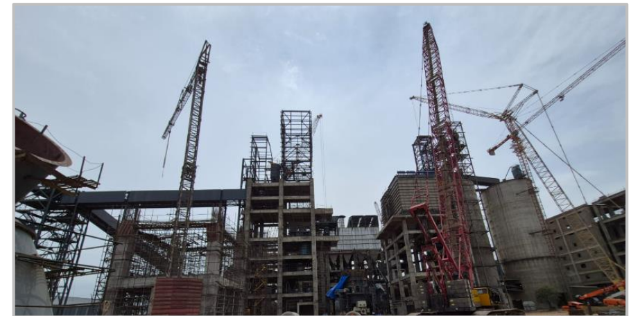
Nagaur IU – Cement Grinding and Packing & Dispatch
