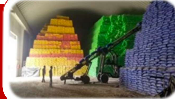
Self-supported roofing structure for a major Indian sugar company at Rajpura, Uttar Pradesh
