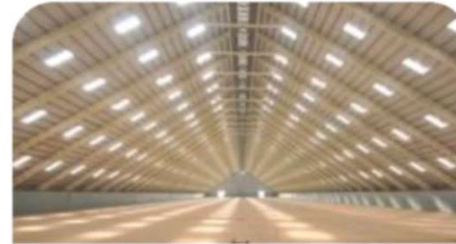
Approx 90,000 sq. m. 'A' frame structure with a centre height of 42 metres and clean span of 84 metres specially designed for the sugar storage requirements for a major Indian sugar company in Kandla, Gujarat
