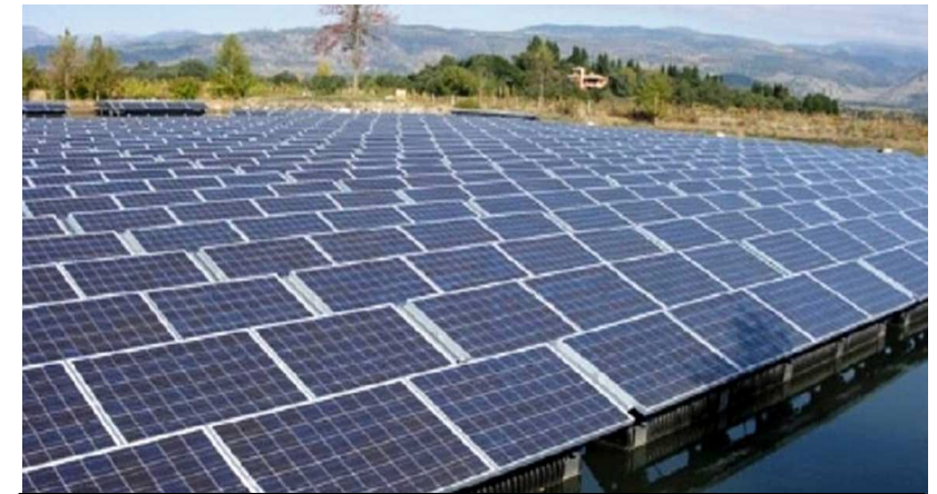
Feeder Solarization Project, Maharashtra
