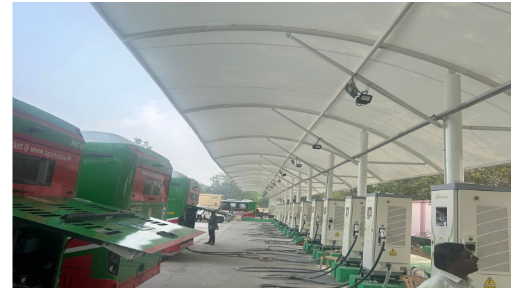
Charging Stations – Telangana
