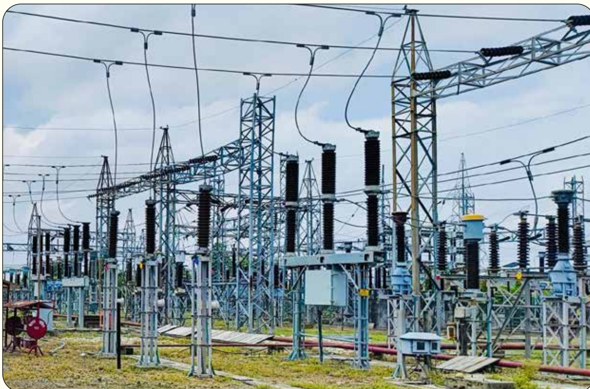
Transformer at the Sub-Station Grid, Dakshin Takmachhara, South Tripura
