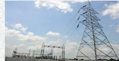
Tower & Substation EPC
