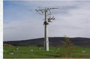
Power Distribution Poles
