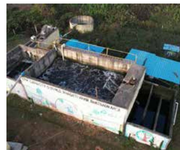
► Mine water treatment plant at SECL
