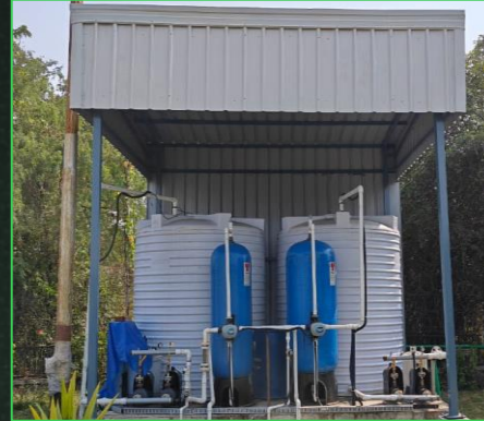
RWH water treatment plant for domestic use
