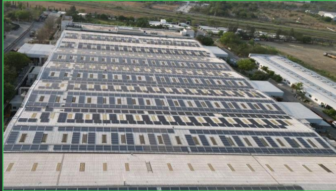
Onsite Roof top Solar system
