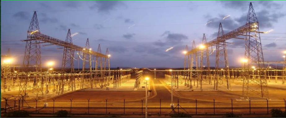
CRP 1 & SAS 2 Solutions
