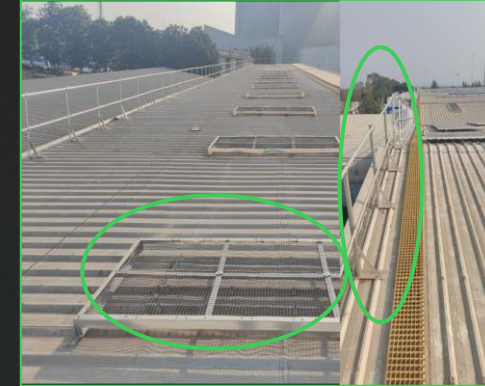
Improved rooftop safety
