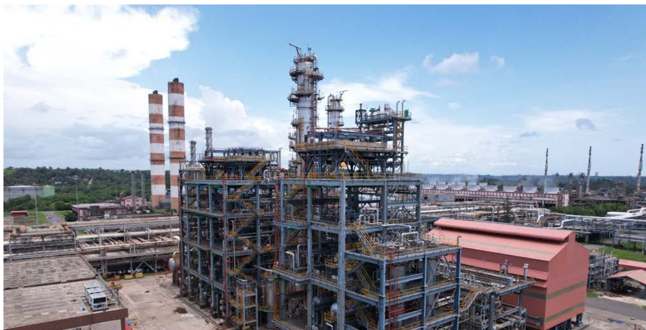
FCC Gasoline Treating Unit
