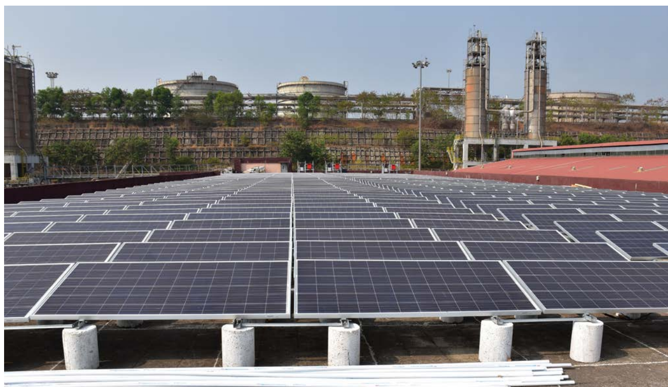
MRPL Solar unit inside the refinery
