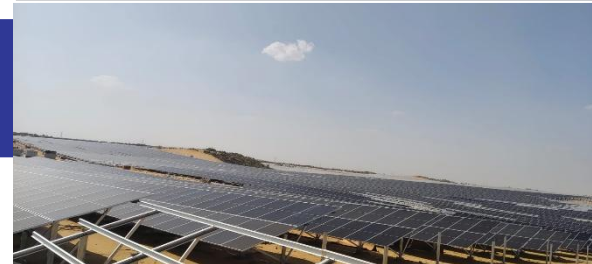
435 MWp Ground Mounted project at Bikaner, Rajasthan
