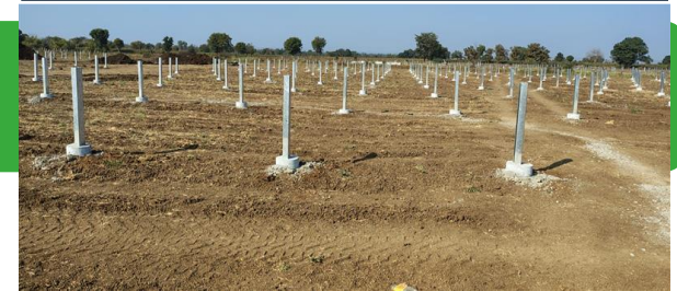
29.4 MWp Ground Mounted project at Yavatmal, Maharashtra
