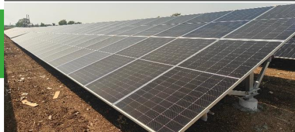
131 MWp Ground Mounted project at Nashik, Maharashtra
