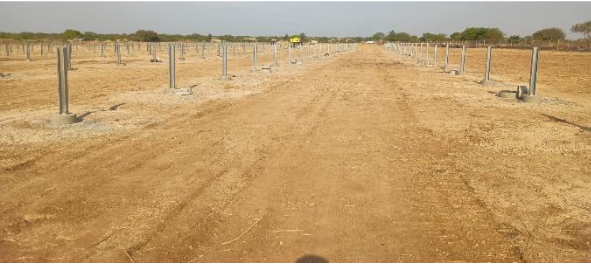
217.5 MWp Ground Mounted project at Solapur, Maharashtra
