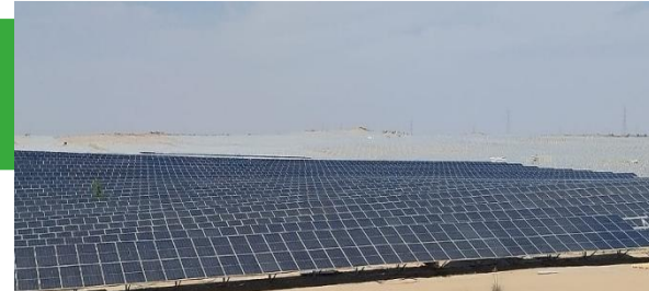
450 MWp Ground Mounted project at Bikaner, Rajasthan
