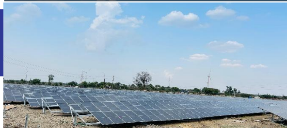
105 MWp Ground Mounted project at Jamnagar, Gujarat
