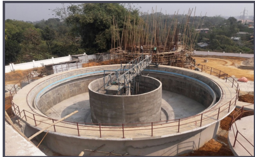
Clariflocculator at Agartala
