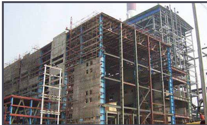
Building and offsite facilities at Unchahar for NTPC
