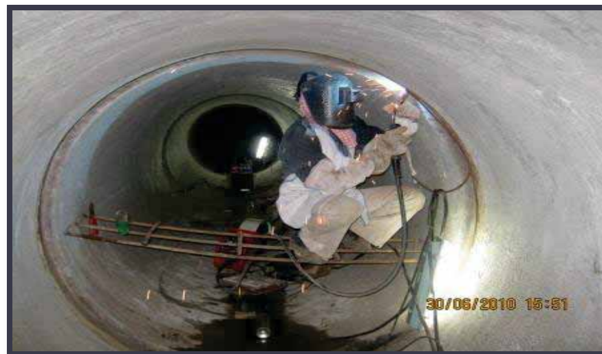
Water transmission line at Tallah Palta
