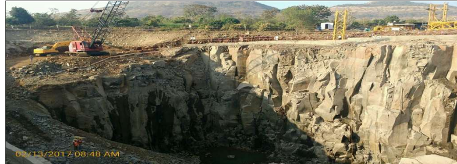
Bhama Askhed Water Supply Project
