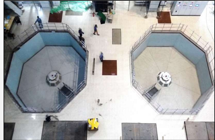
Power House, Umtru
