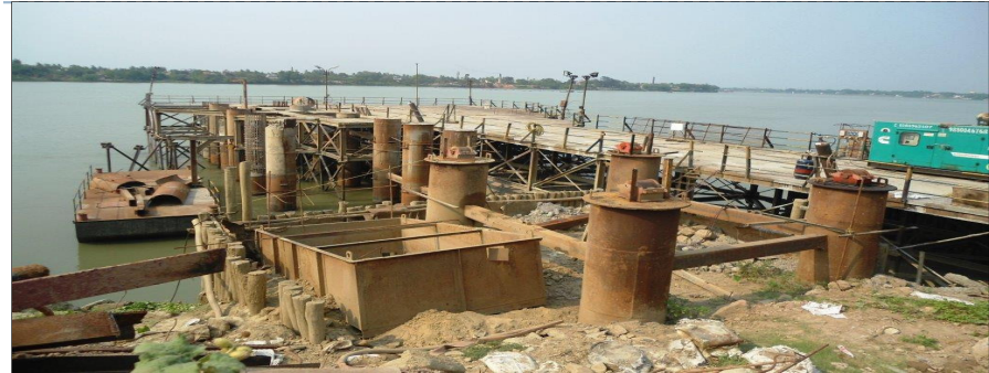
Intake jetty at Palta WTP, Kolkata
