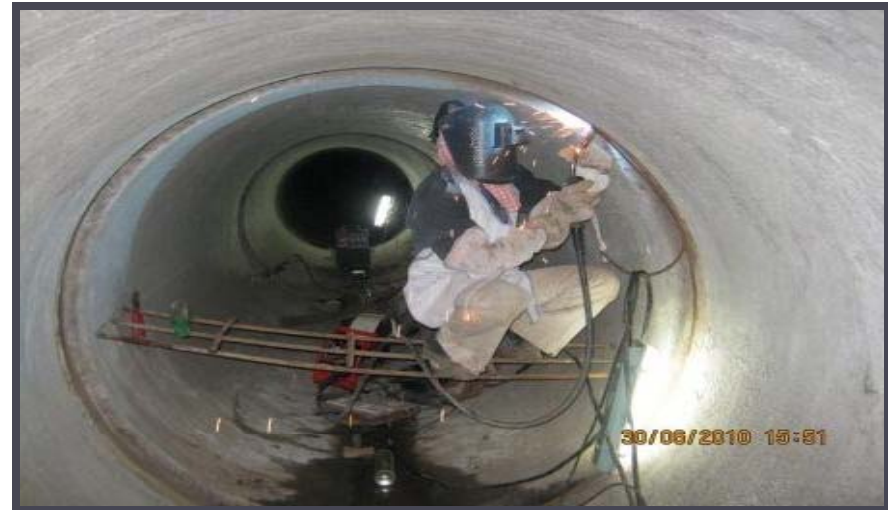
Water transmission line at Tallah Palta
