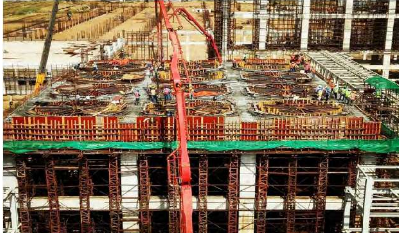
Paradip Refinery – Industrial Complex
