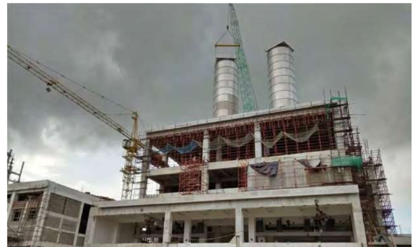
Paradip Refinery – Industrial Complex
