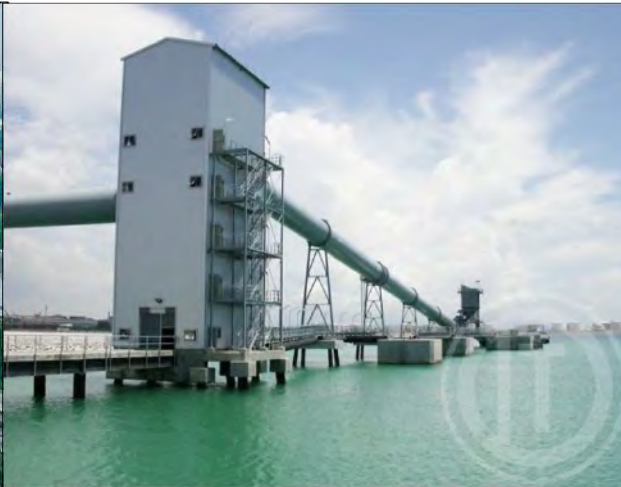
COCO Coal Handling System
