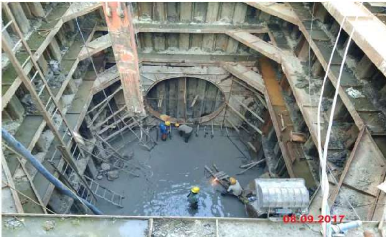
Trunk Sewer KEIP
