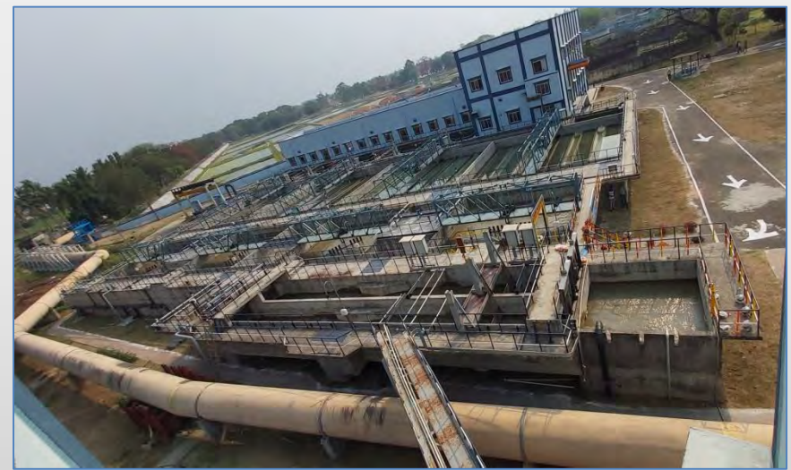
Palta WTP, West Bengal
