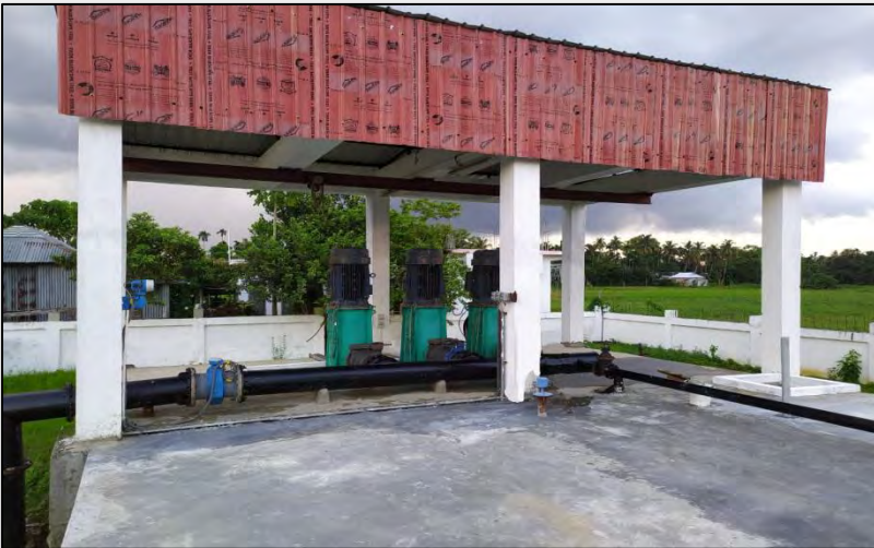
Clear Water Pumps at Rampur, Agartala
