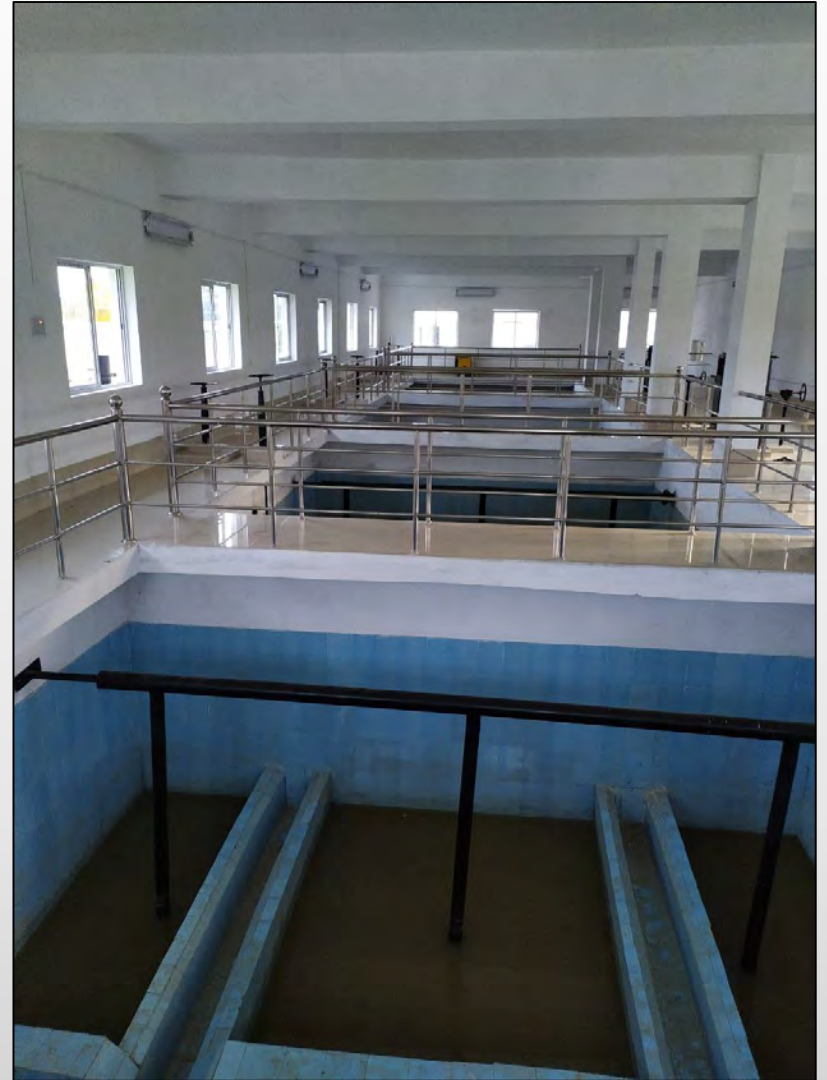
Filtration Plant at Rampur, Agartala
