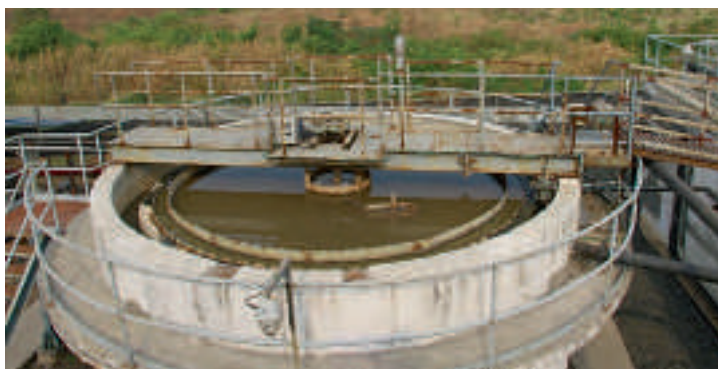
Water Treatment Plant at our Ambarnath manufacturing plant
