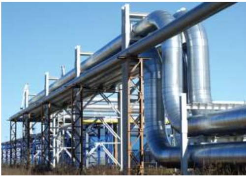
NTPC IVRCL, Main Plant, Allahabad
