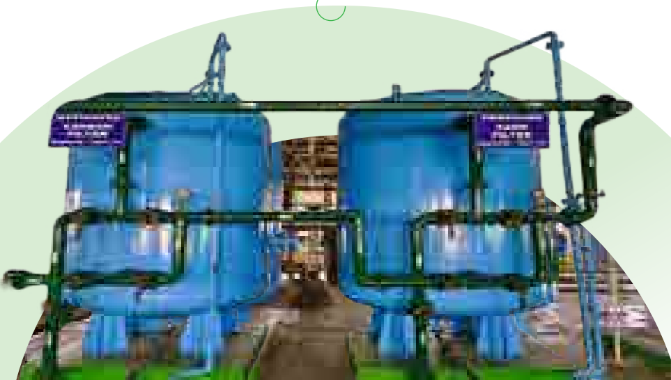
Rain Water Harvesting Tanks at Hosur Plant
