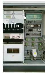
Continuous Emission Monitoring System
