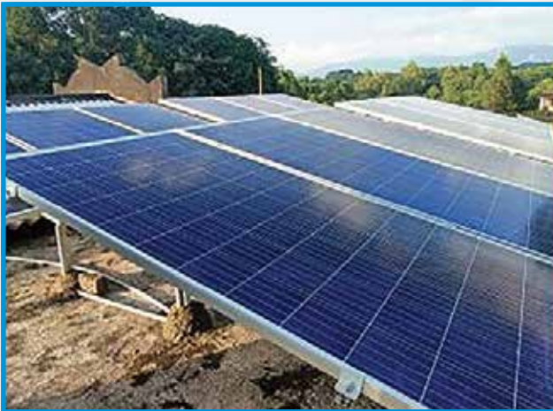
▲ Rooftop solar panels installed
