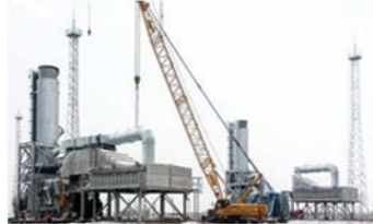
35 MW GT POWER PLANT, KAZAKSTHAN
