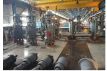
CONTROL & STOP VALVES OVERHAULING SIPAT 660MW
