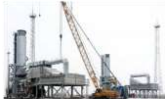
35 MW GT POWER PLANT, KAZAKSTHAN
