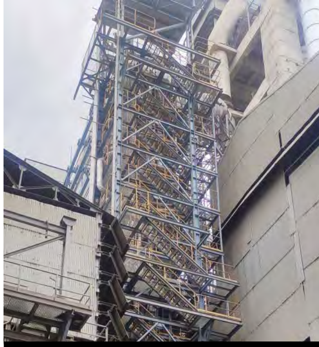
P H Boiler
