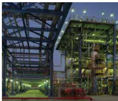
Left: Rajasthan: Raageshwari Gas Terminal
