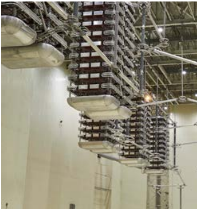
Valve Hall 765 kV HVDC at Kurukshetra
