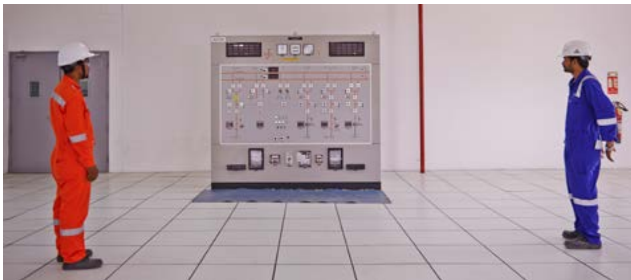
Grid Automation Unit - Pallavaram
