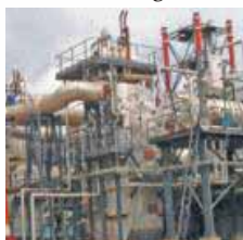
Tank Farm heating
