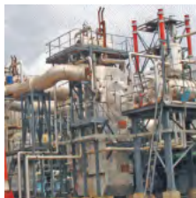
Tank Farm heating
