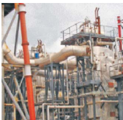
Tank Farm Heating
