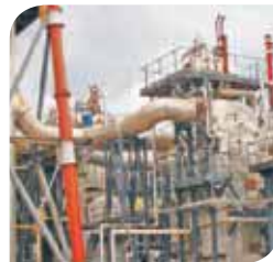
Tank Farm Heating
