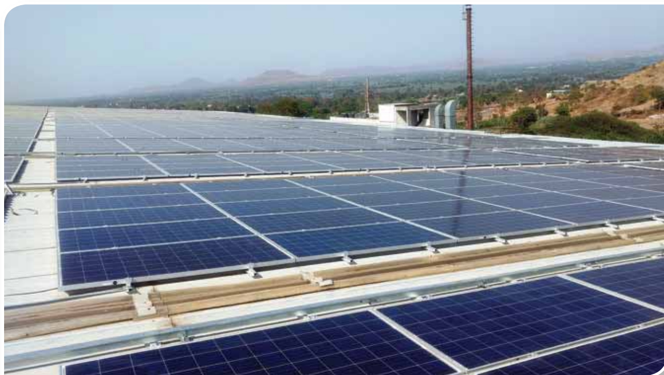
Thermax's solar installation for a major auto ancillary in Maharashtra. It has a capacity of 850 KW with an estimated generation of 1.2 million kWh/annum and will help reduce 983 tons of carbon every year. The installation has net metering to feed excess power to the Maharashtra state electricity grid.
