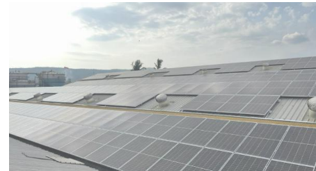
Rooftop Solar Panel
