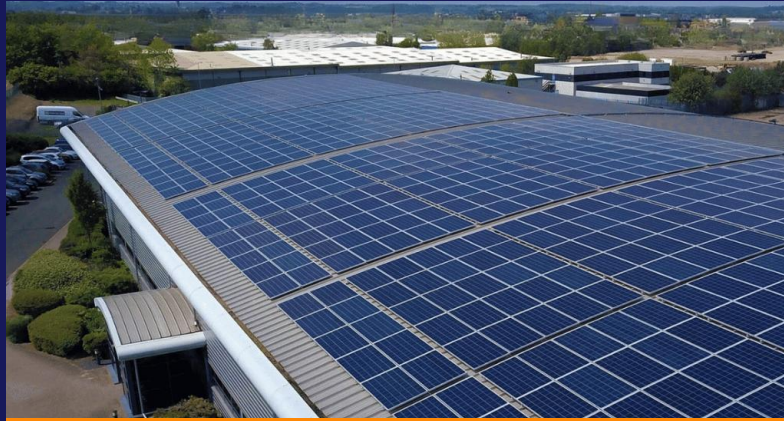
Solar Industrial Rooftop
