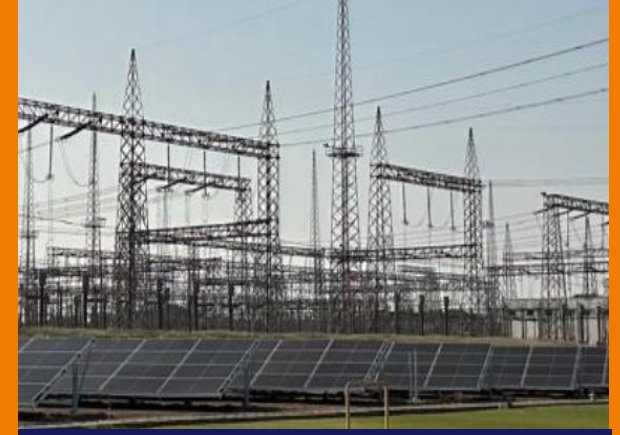
Torrent Power Ltd (3.0 MW) Surat, Gujarat
