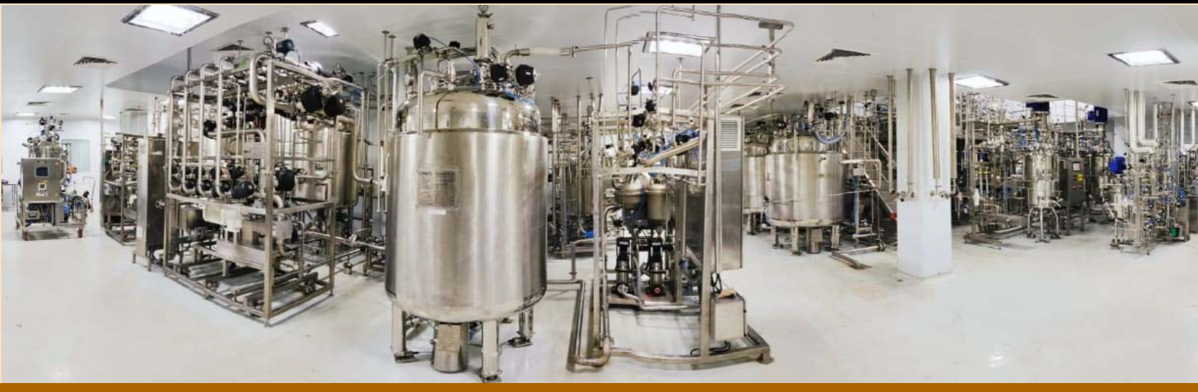
Microbial Products Upstream Facility
