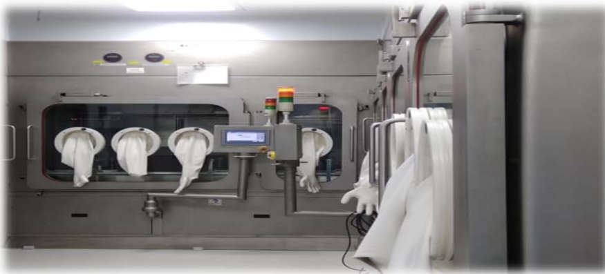
Filling facility – Fully Automated
